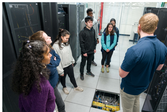
Figure 2: Adam Carlson highlighting the raised flooring and cabling of the WFU Data Center during a tour with students. Photo credit: Sean M. Anderson.
